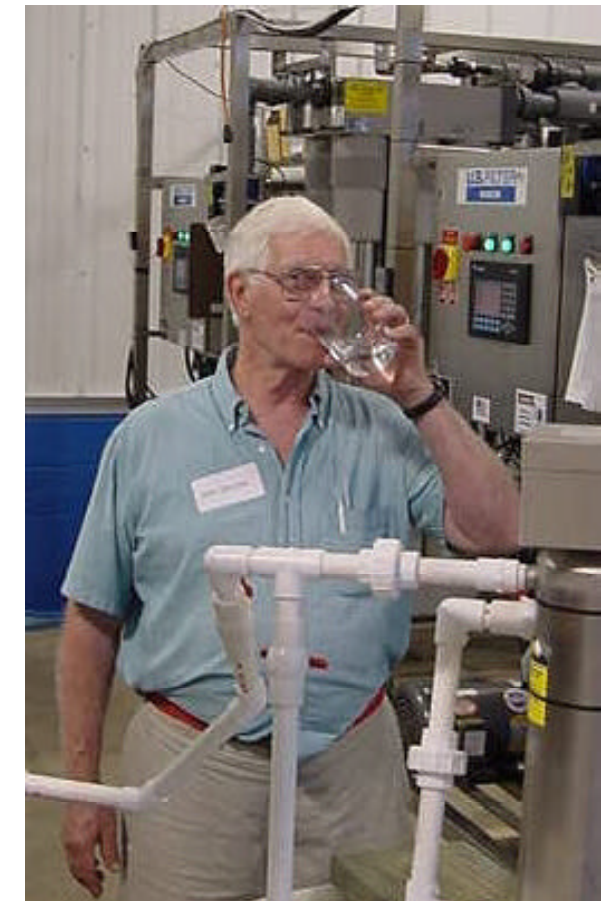
John lines up for a drink of recycled water from UAJA's Beneficial Reuse project. Wastewater is treated to drinking water standards to be reused by the community and eventually recharged into the groundwater aquifer in the Slab Cabin Run watershed.
